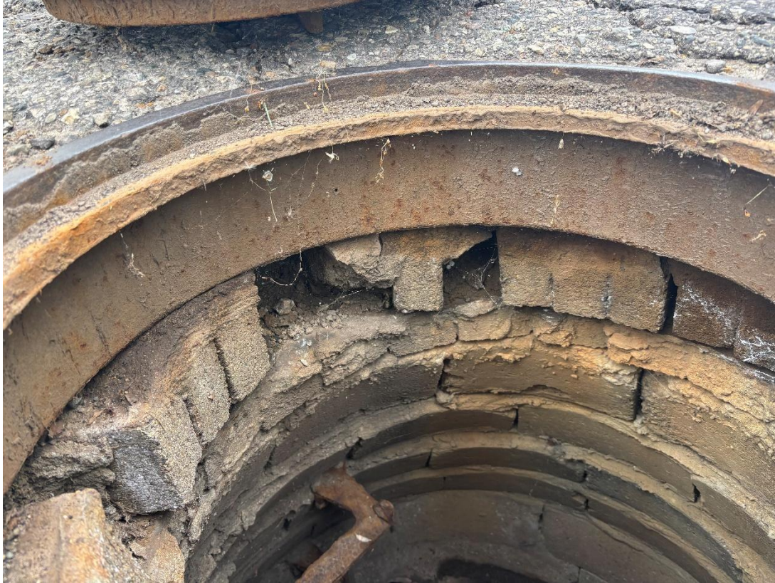
Sanitary Manhole SS1472 – Photo 3, chimney/casting issues
