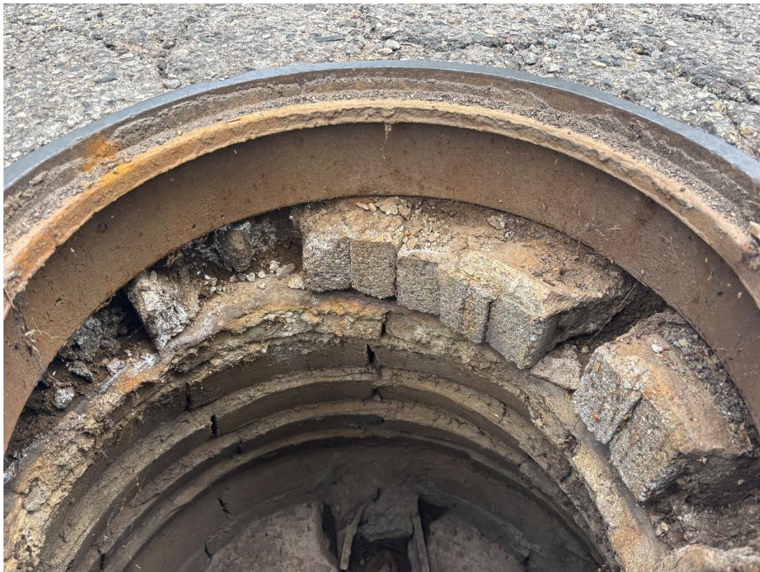
Sanitary Manhole SS1472 – Photo 4, chimney/casting issues
