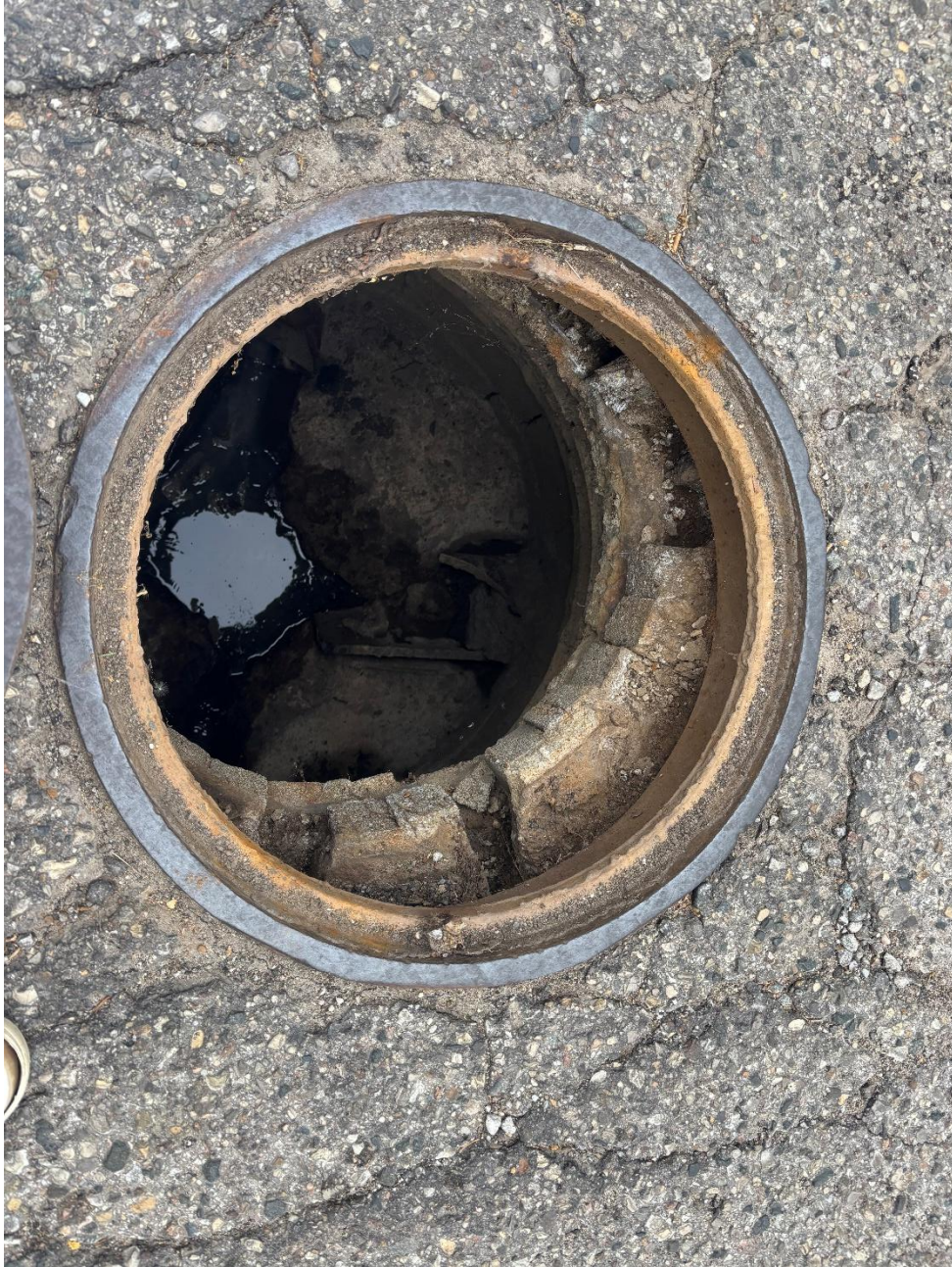
Sanitary Manhole SS1472 – Photo 1, chimney/casting issues
