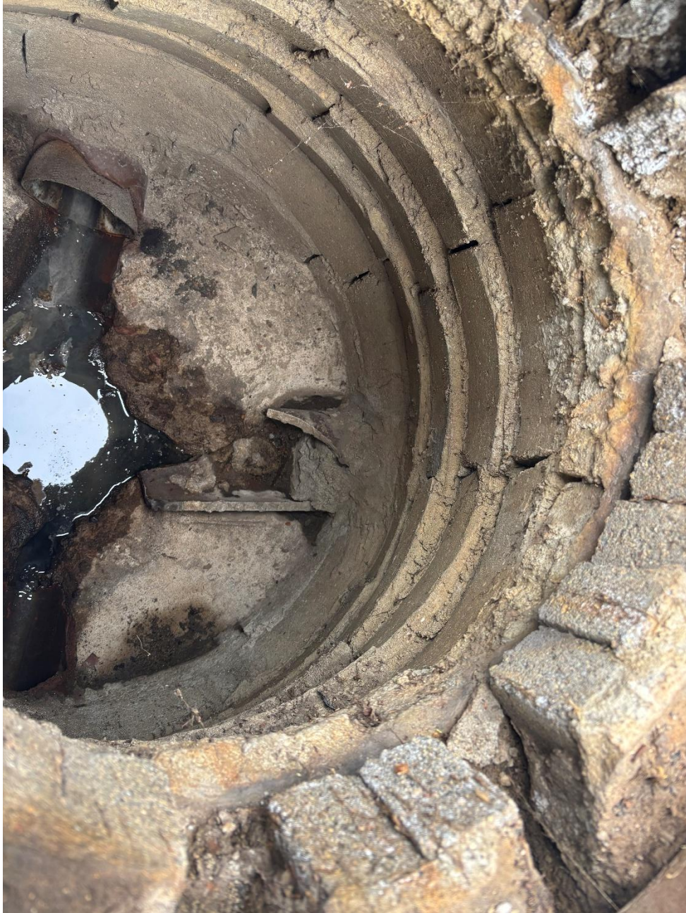
Sanitary Manhole SS1472 – Photo 2, chimney/casting issues
