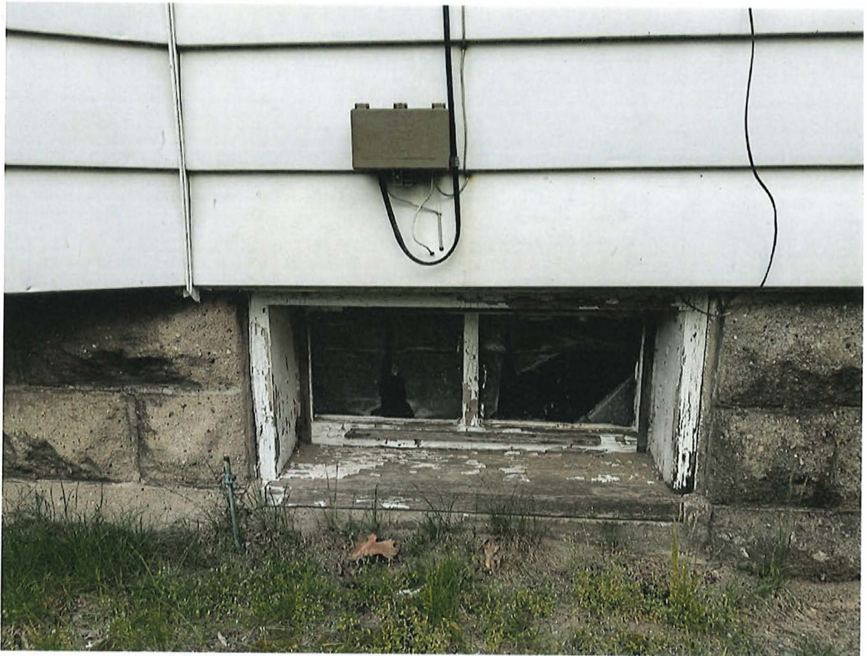
Photo: 4" Basement window at the back of the house is obscured by the trash can.
